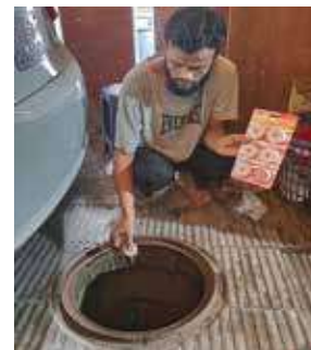
Water Meter hole
